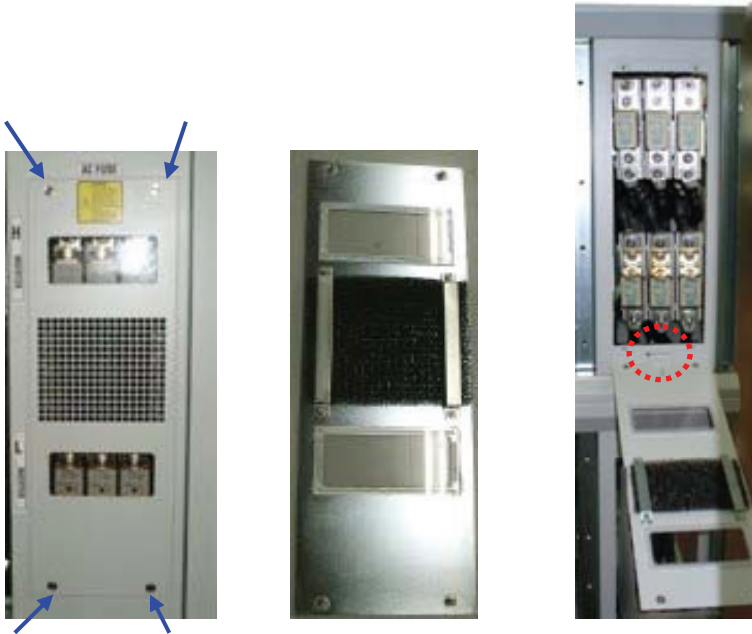
Figure 15-6- “DC Fuses Zone” (the inside and the outside of the panel)
