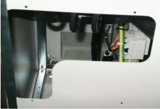
Figure 11-2 : Opening for DC wires between Frameworks – seen from below.
