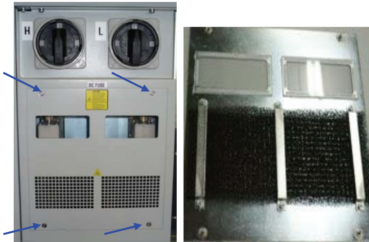
Figure 15-4- “DC Fuses Zone” ( the inside and the outside of the panel)
