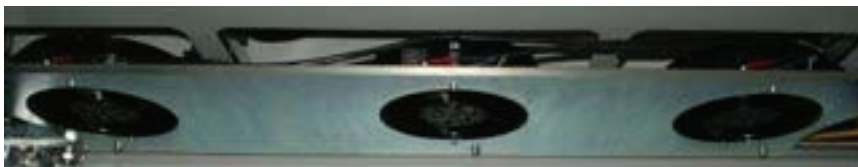
Figure 15-8: Position of the fans in the ACBOX compartment
