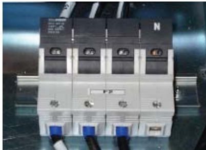
Figure 15-11- F2 fuse box for OVR AC protection
