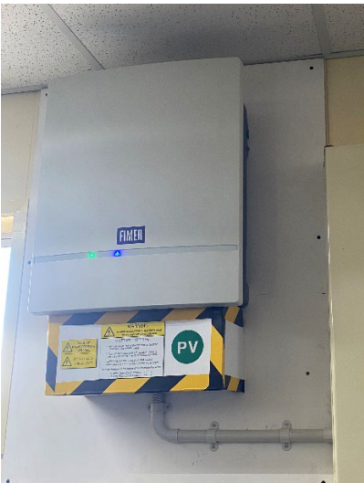
Image – FIMER's PVS-15 installed and commissioned by Egmont Solar.
