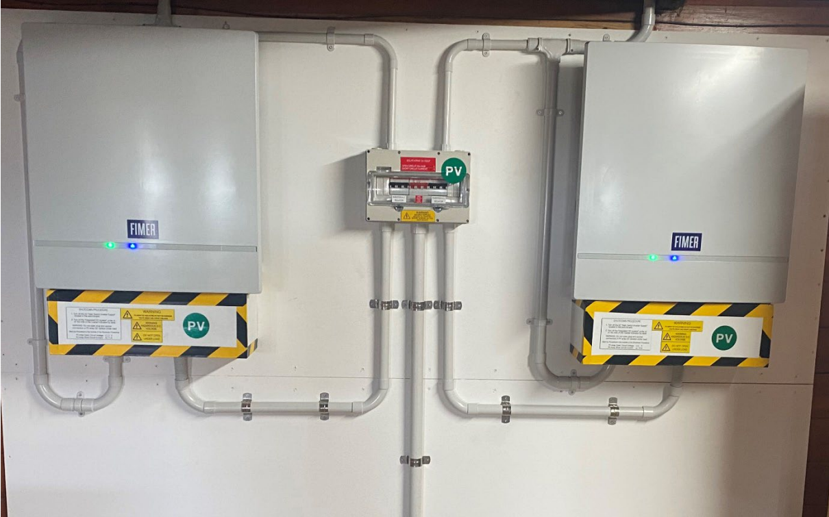
Image above- Two of FIMER's PVS-20 installed and commissioned by Egmont Solar.
