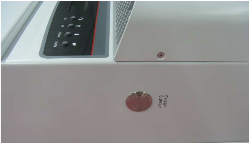
Fig. 18 – Button for starting-up the inverter from the grid
